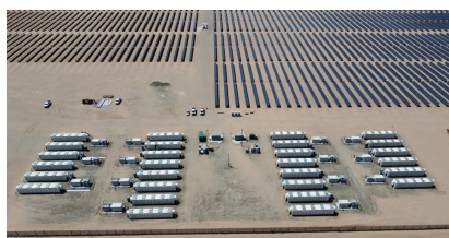
Invenergy's Foothills Storage Energy Center in Yuma, Arizona
