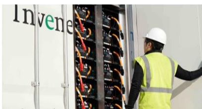
Storage at Invenergy's Grand Ridge Energy Center in LaSalle County, Illinois
